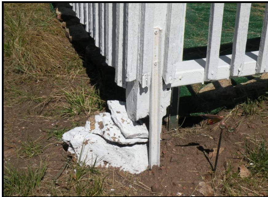
Figure 58. The deteriorated base of a grave enclosure corner post has been replaced by a channeled metal rod and natural stones, painted white.
