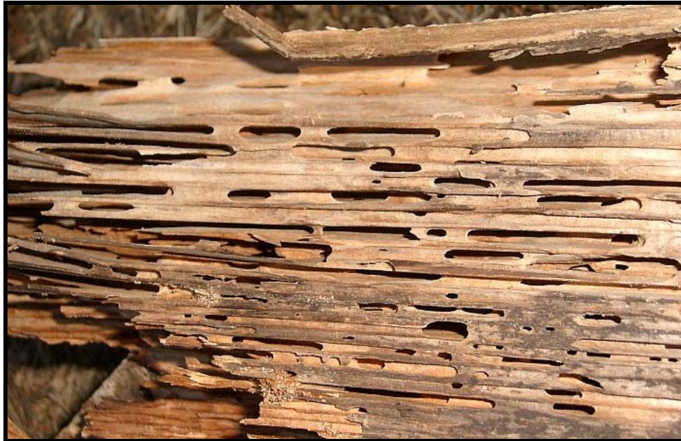
Figure 29. A wood truss with severe carpenter ant damage (Fritsche 2005).
