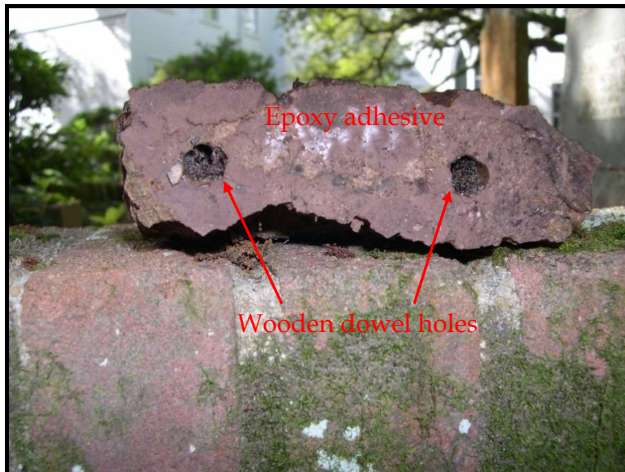
Figure 52. The repaired end of the marker (from Figures 49, 50, and 51) shows that the epoxy remains but the wooden dowels have rotted away.
